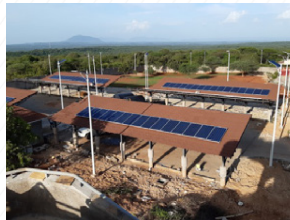
30KW Solar project at the Hydro plaza
