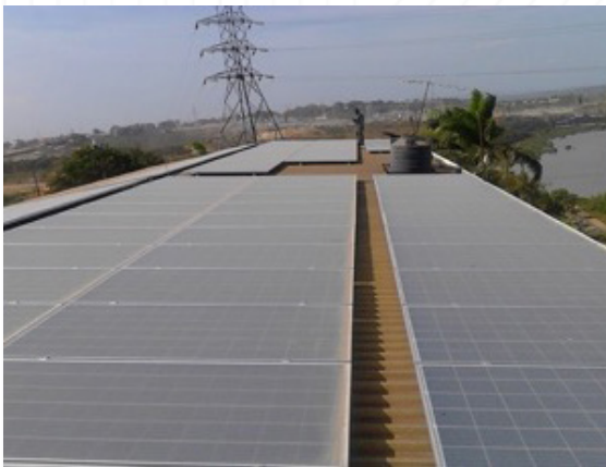
40KW Solar project at Kipevu power station
